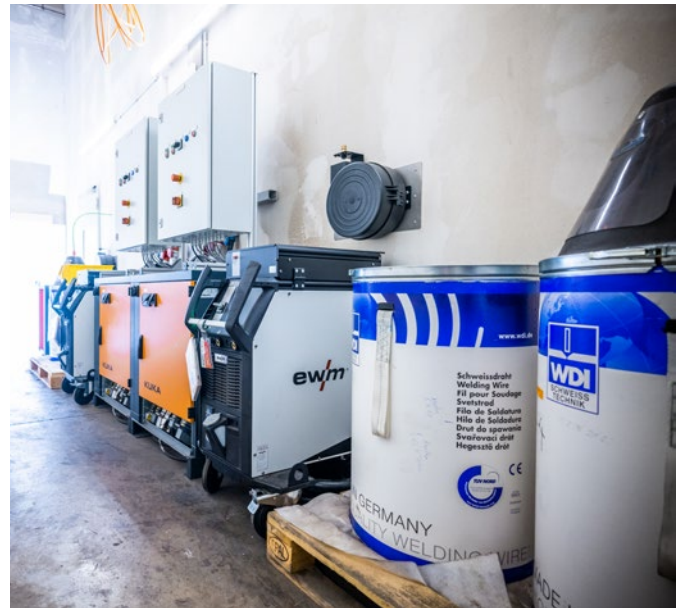
The system control, welding machines and filler material in the drums are located behind the rear panel of the welding booth to prevent exposure to soiling.
