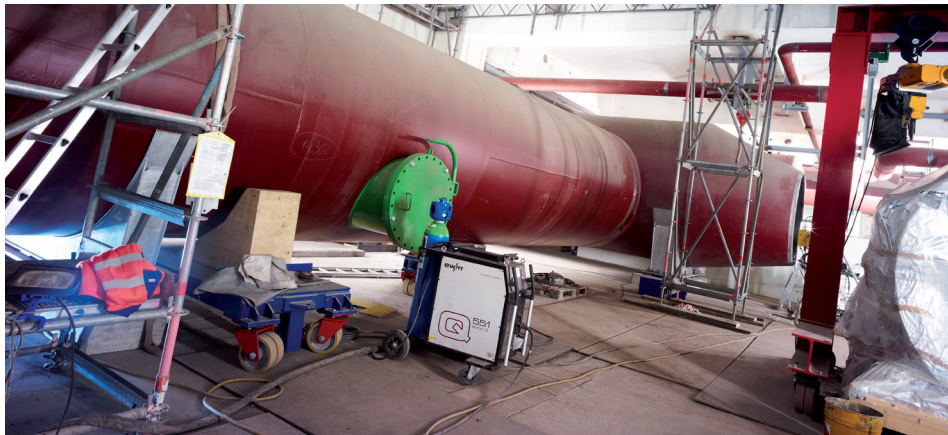
/ Coolant water pipes with diameters of up to 3,400 millimetres – welded segment by segment for precision – are constructed using the TÜV Hesse-certified MAG process for the first time
