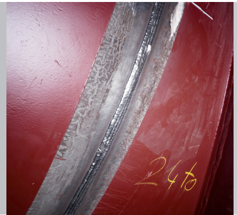
/ Perfect MAG welding in one operation – the program-controlled, reduced energy pipeSolution® process produces the required weld pool viscosity in any position
